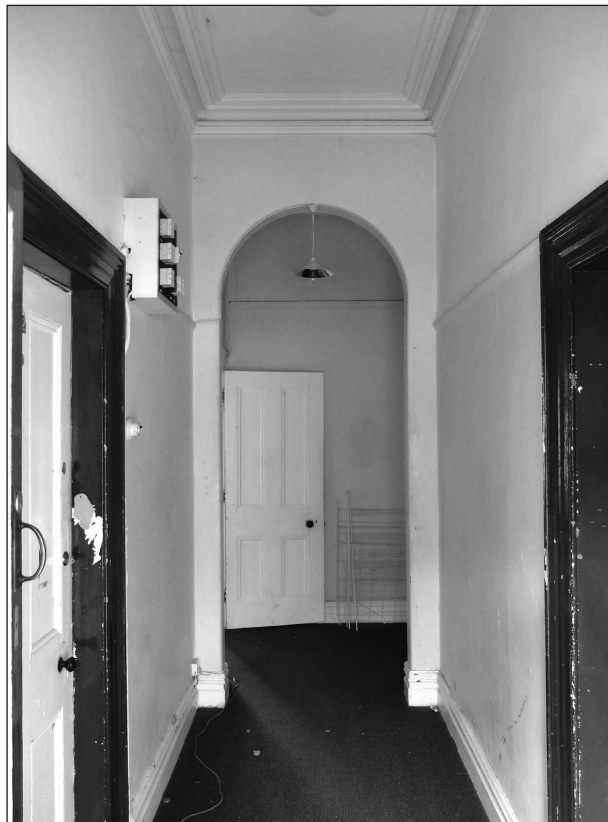
Figure 10. The main upstairs hallway, with the original lath and plaster lining in place from floor to ceiling, and the original architraves, skirting boards and ceiling cornice intact.
