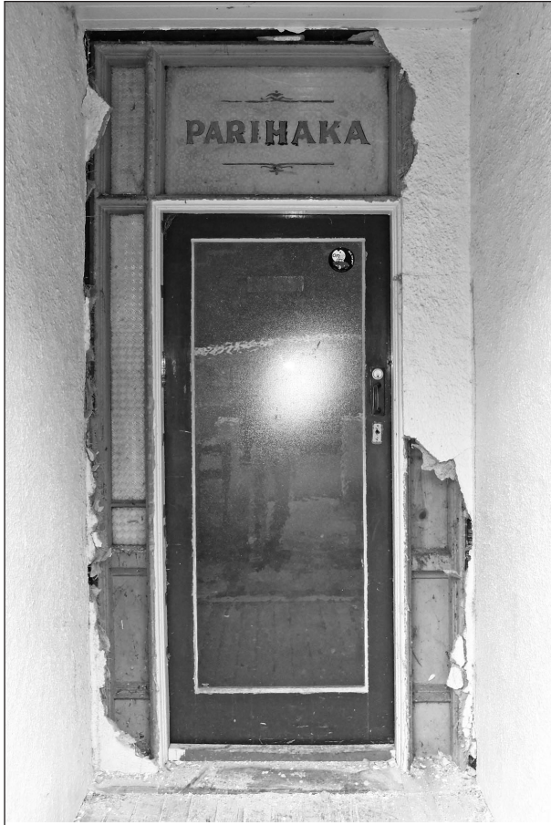
Figure 6. The front door of 29 Queen Street as the 1940s stucco was stripped back to reveal the original 1880s door frame and 'Parihaka' fanlight.
