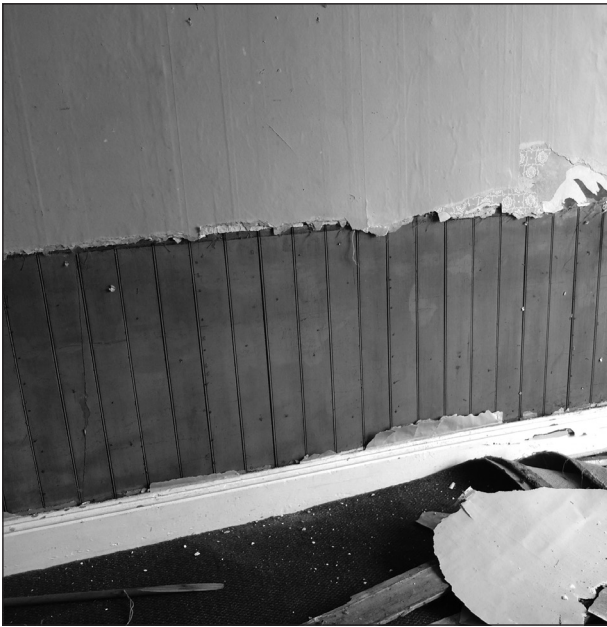
Figure 14. The timber wainscot revealed in the downstairs north-east room (Room 7) during stripping of the wall linings.
