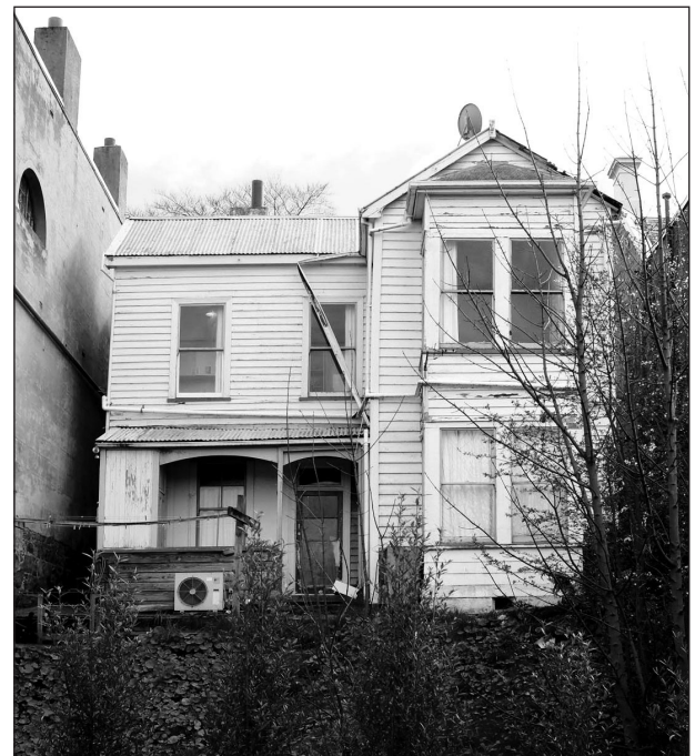
Figure 8. The rather decrepit rear elevation of 29 Queen Street in 2015, with missing bargeboard, failed guttering and decayed weatherboards. However, the formal aspect of this elevation is still apparent.
