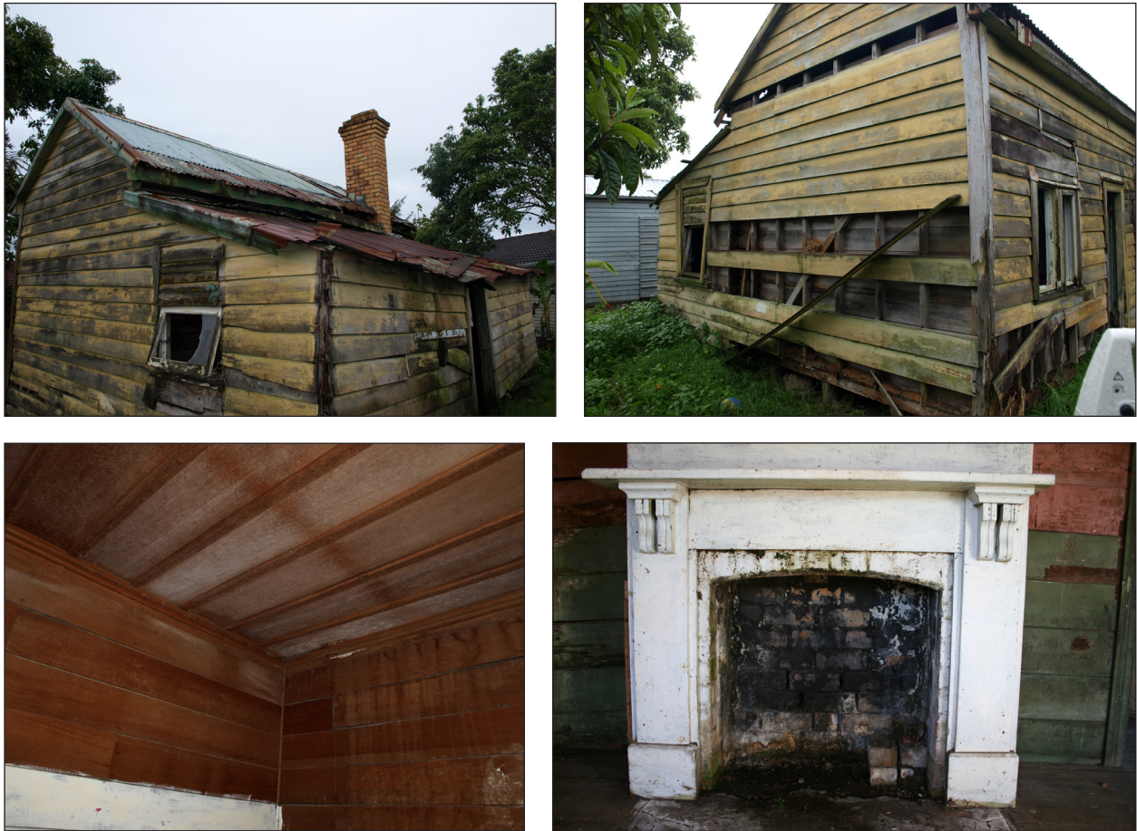
Figure 4. The cottage at the time of investigation: top left, the south west corner; top right, the north east corner; bottom left, the walls and ceilings of Room 2; bottom right, the fireplace surround in Room 1.
